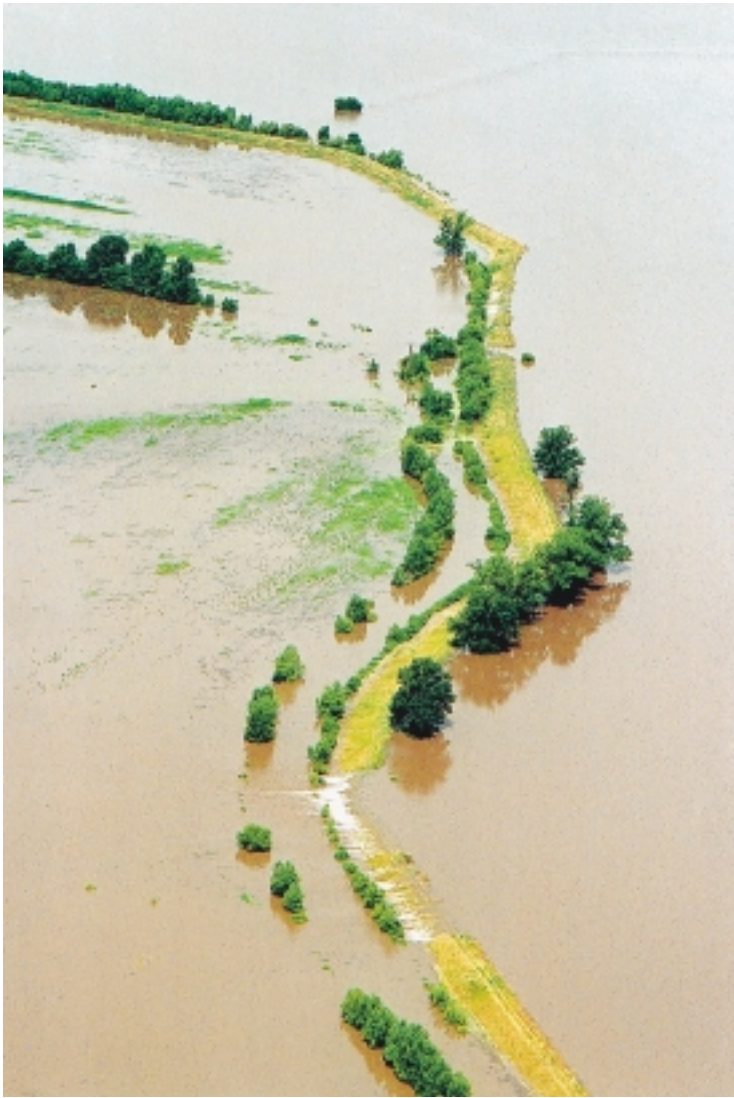
Figure 15-11. Levees were damaged in two ways: from being overtopped as shown here, or from seepage. In either case the levees usually were eroded by the force of the water through the restricted space. Large, deep holes were scoured in the Unimpounded Reach and the Missouri River (Source: St. Louis Post-Dispatch ).
